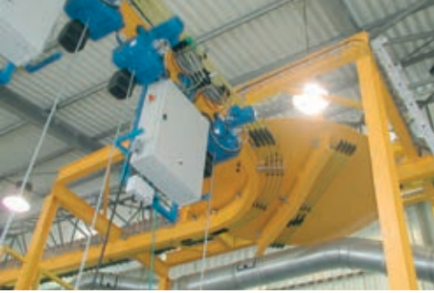
SinglePowerLine 0812 in a galvanizing plant with bridge elements on a turning gate and dual collector assemblies
