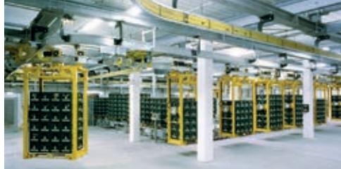
SingleFlexLine 0811 on an electrified monorail system in a brewery
